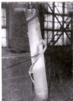
图10 涂料剥脱良好 Fig.10 The paint peeling well
