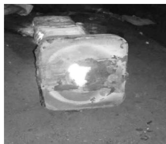
(c)严重破损
